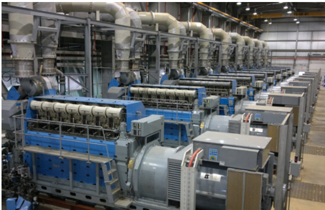
Ambatovy power plant with 9 × 7L27/38 is located on Madagascar.
